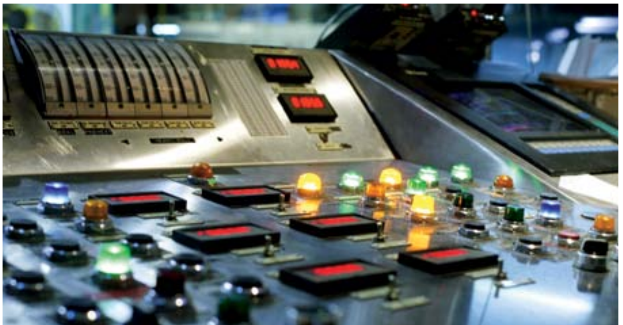
■ Sorevco operates 24 hours a day, seven days a week. To have a broken crane means severe production loss.
